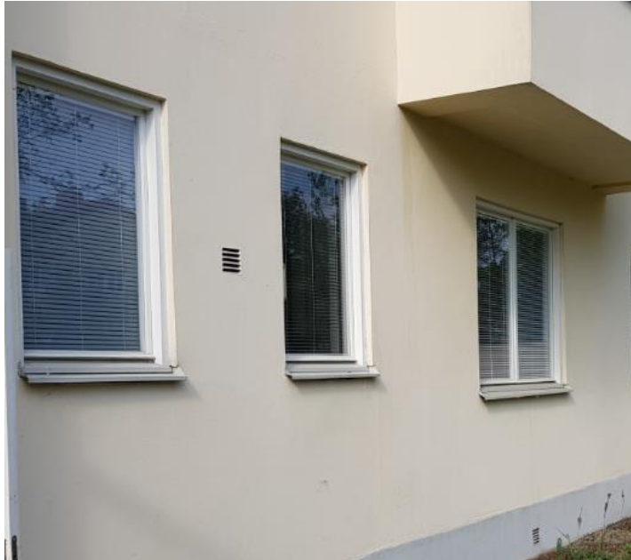
Figur 2. Fasad i ok skick.
